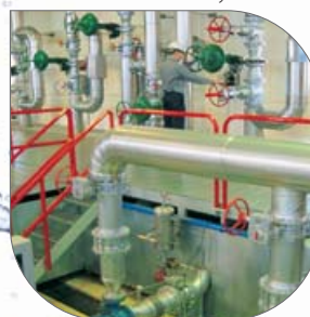
<< Industrial Process Systems
